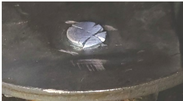
This is the flattened bolt end in the window regulator arm.
